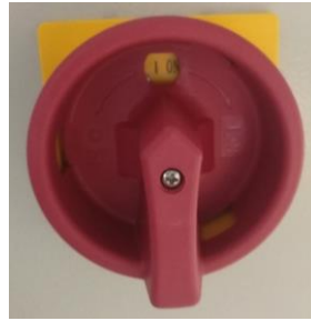
Master switch (ON)
